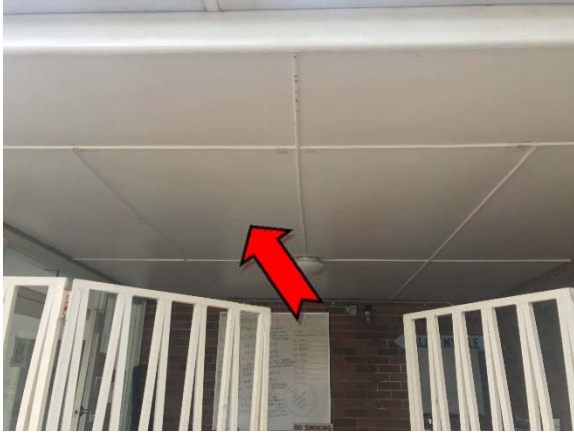
Photo 1. Exterior, throughout, awning – asbestos-containing fibre cement sheeting.
